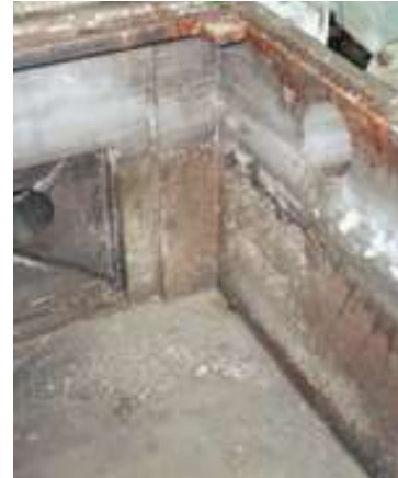
Corrosion in the resevoir
